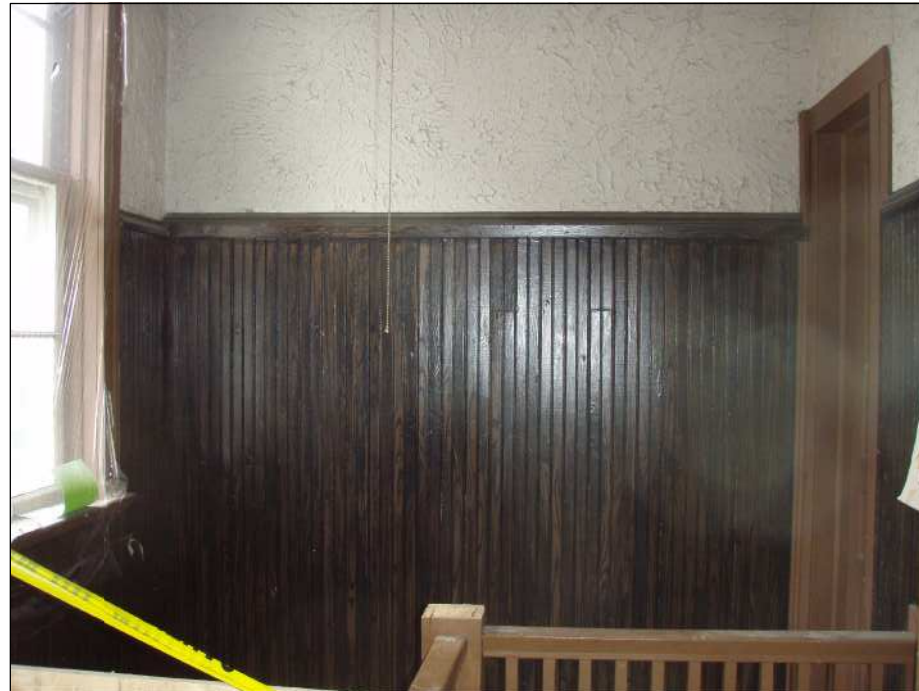
- EXISTING WOOD WAINSCOT PANELS. - NEW WAINSCOT, WOOD WALL BASE AND TOP RAIL TRIM TO MATCH SIZE, STYLE / PROFILE AND DIMENSIONS OF EXISTING PANELS.
