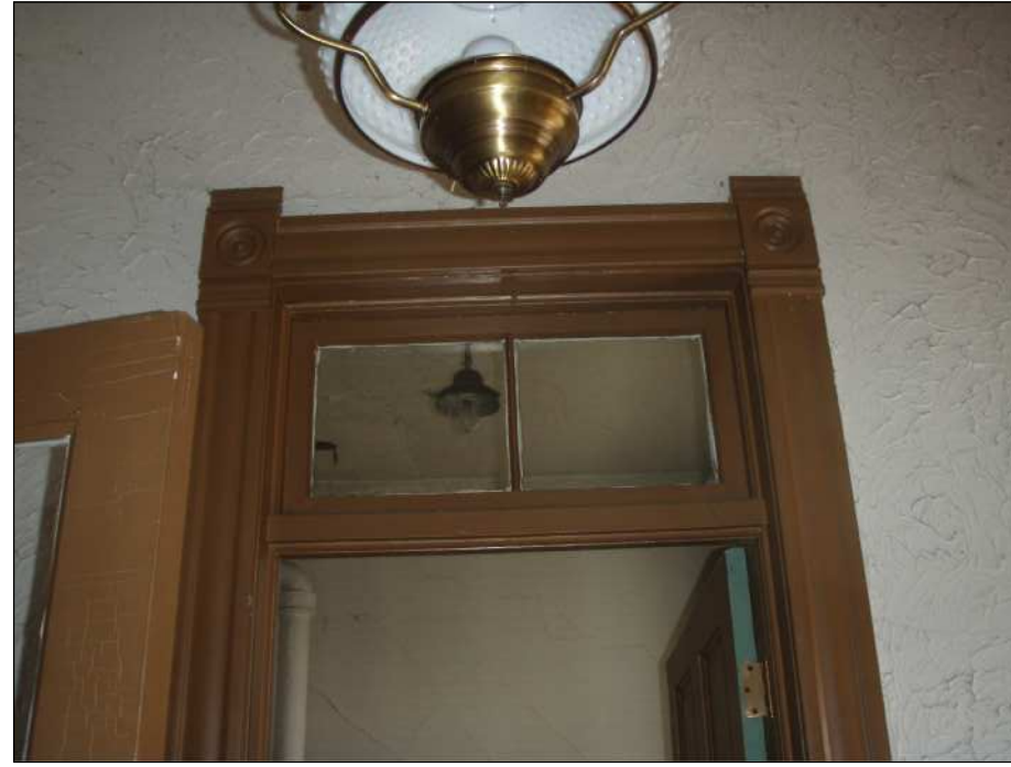
- EXISTING WOOD ARCHITECTURAL TRIM AND TRANSOM TO REMAIN. SURFACES TO BE PREPARED TO RECEIVE PAINT. - NEW DOORWAY AND TRANSOM ON OPPOSITE WALL TO MATCH SIZE, STYLE AND DIMENSION OF EXISTING.
