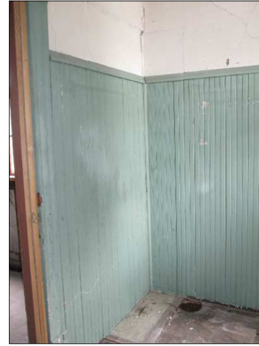
- EXISTING WOOD WAINSCOT PANELS. - NEW WAINSCOT TO MATCH SIMILAR SIZE, STYLE / PROFILE AND DIMENSIONS OF EXISTING PANELS.
